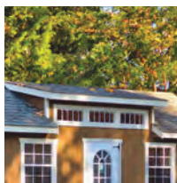
Shed Dormer w/Broken Roofline*
